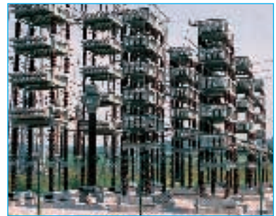
High Voltage Capacitor Banks
